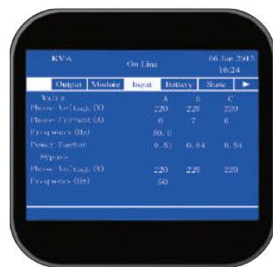
UPS Cabinet Control Panel
