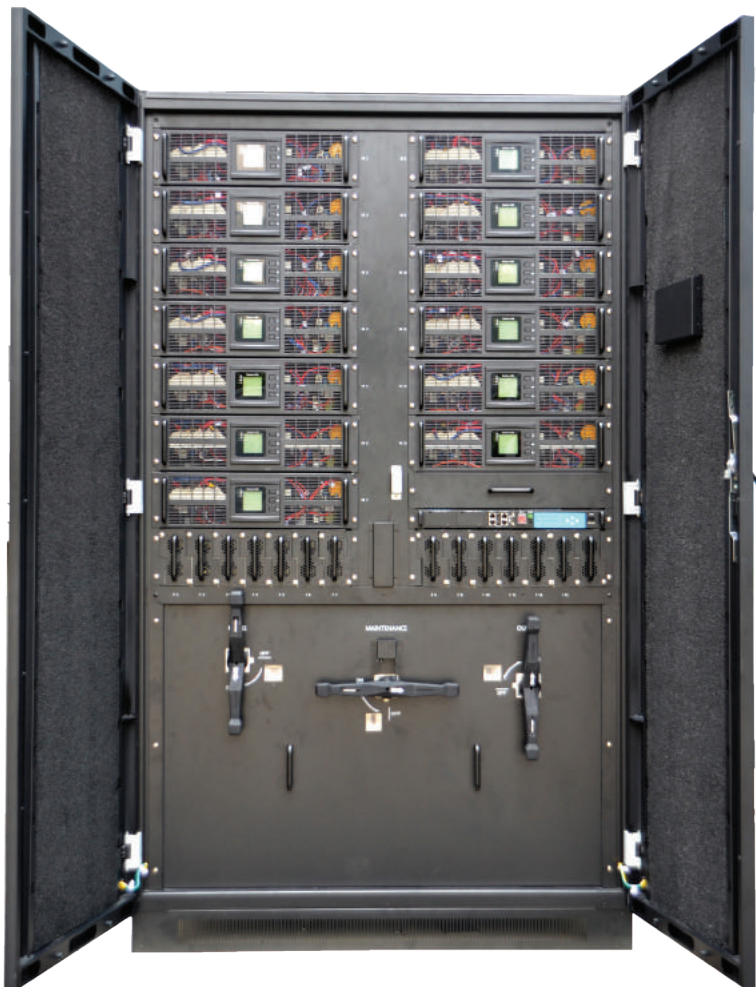
520kVA cabinet (13x40kVA) .
